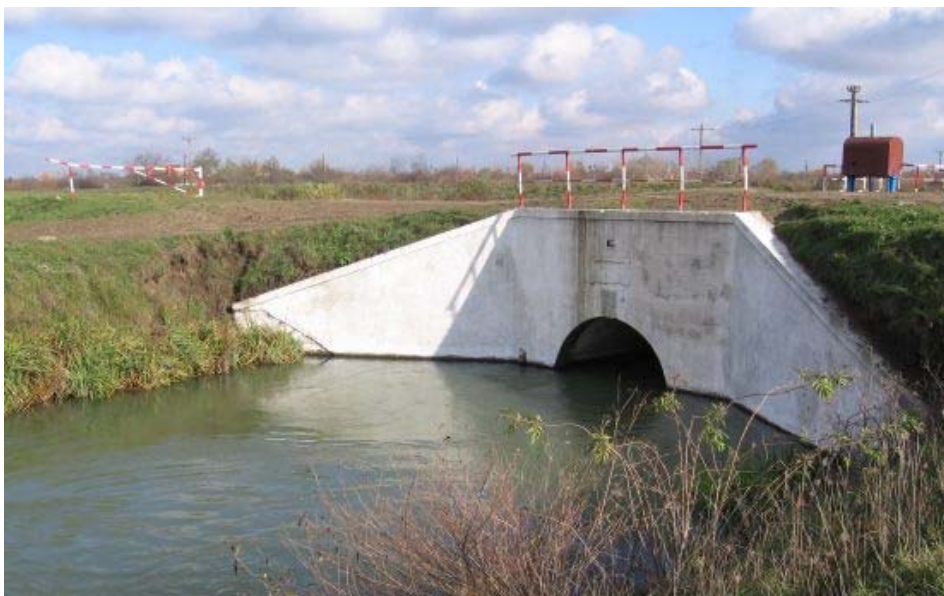
Fig. 2. One of the weirs of the Collector channel.
